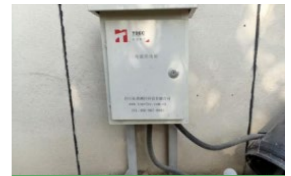
Jiangxi Ya Dong has implemented round-the-clock real-time monitoring of blasting vibration in its mining area.
